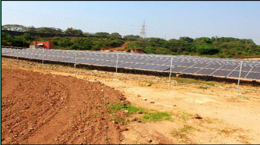
[View of 1.3 MWp Solar Plant at BFU premises of KIOCL at Mangaluru]
