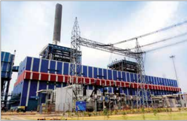
2x270 MW Adhunik TPS-Unit 1 commissioned
