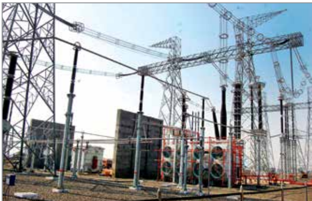
1200 kV Transformer at PGCIL Test Station at Bina
