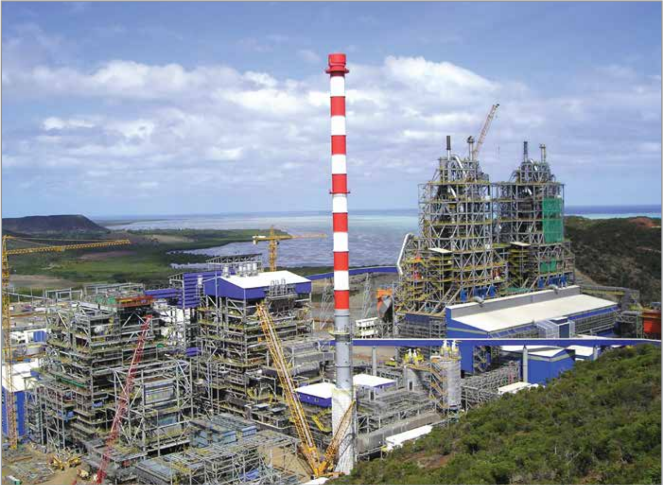
Two nos. 135 MW Circulating Fluidised Bed Combustion (CFBC) Boilers under commissioning at New Caledonia
