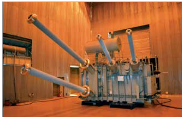
498 MVA, 500 kV Converter Transformer for \pm 500 kV, 2500 MW Balia-Bhiwadi HVDC project
