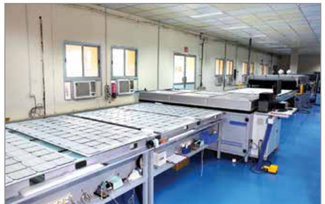
New Automated Solar Photovoltaic Panel manufacturing facility at EDN, Bengaluru
