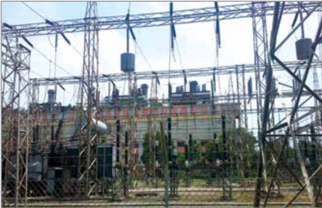
110 MW Unit uprated to 120 MW by BHEL at PSPCL GNDTP Bathinda TPS-3
