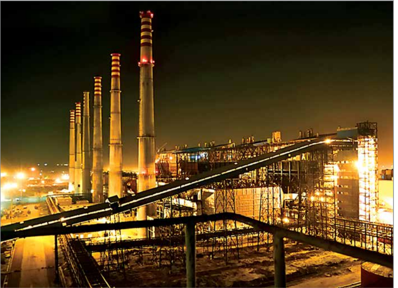
BHEL's first two-cylinder uprated 150MW (Reheat) rating turbine in the Industrial Segment commissioned for HINDALCO at Mahan
