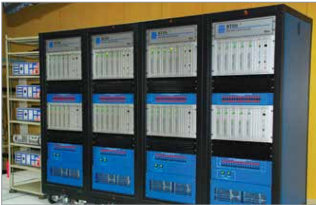
Real Time Digital Simulation Facility installed at COE-ATS at Corporate R&D
