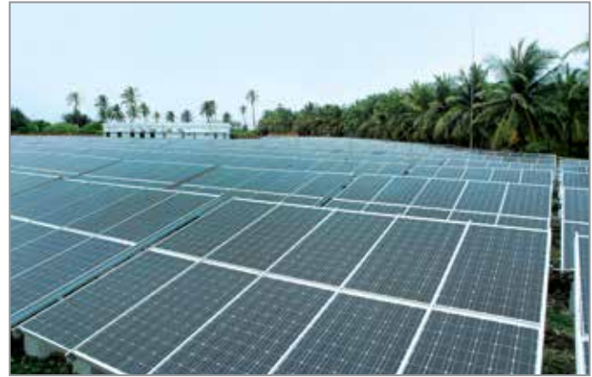
Grid Interactive Solar Power Plant-commissioned a total of 1.9 MWp SPV plants at various islands of Lakshadweep for the Deptt. of Electricity
