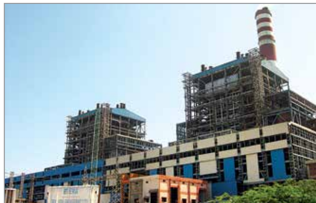
2x600 MW North Chennai TPS-commissioned India's first indigenously manufactured sub-critical set of 600 MW on EPC basis
