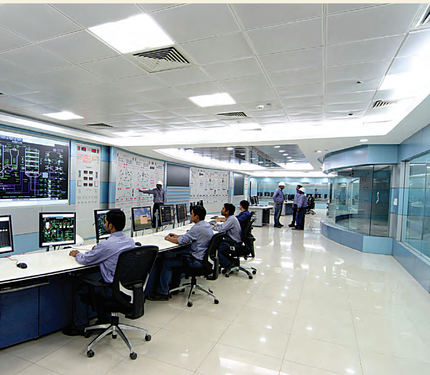
Control Room at the Vijayanagar power plant
